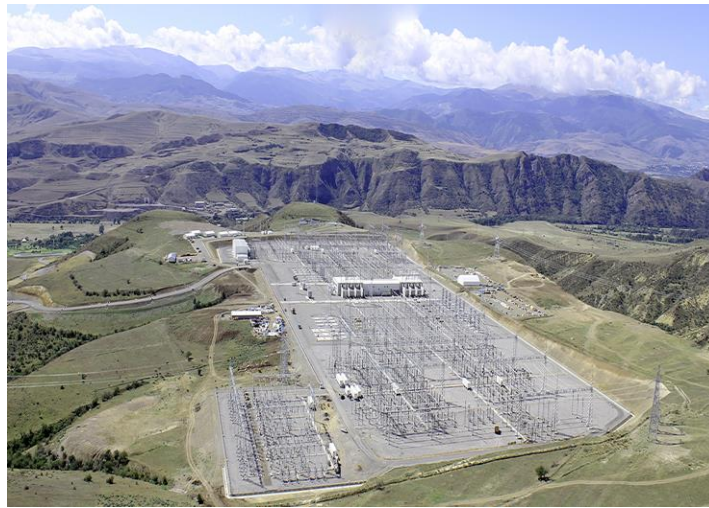
Fig .3. Akhaltsikhe 700 MW and 500/400 kV High Voltage Direct Current (HVDC) plug
